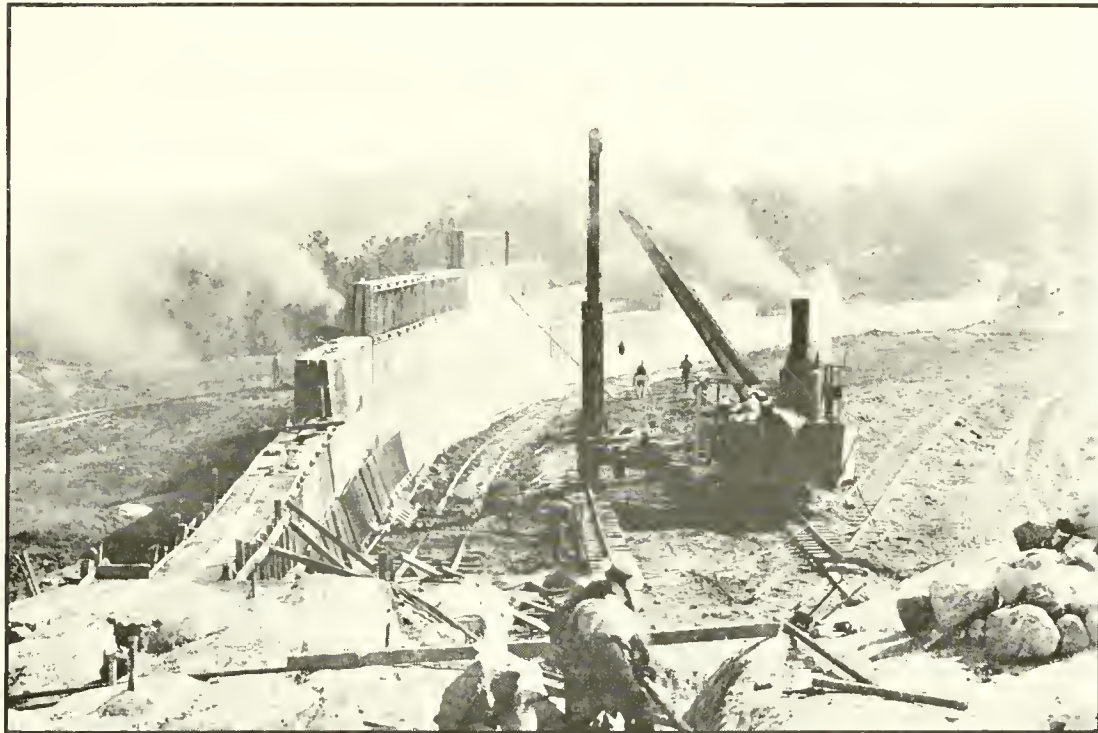
Phelps Brook Dam, Being Built by The Pierson Engineering Co. of Hartford, Conn.
