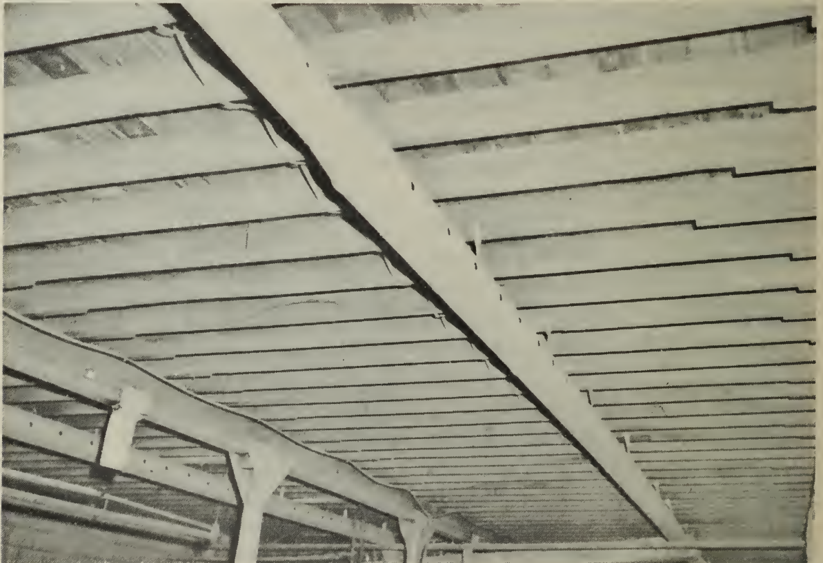
Figure 25. A broiler house in which tempered air is brought from a hot-air furnace and distributed through round pipes to aid ventilation.
