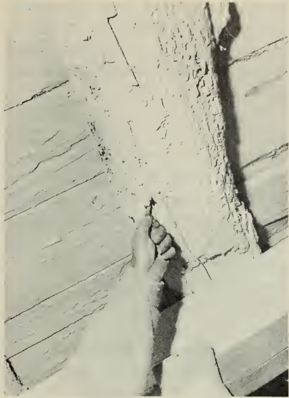
Figure 1. A beam in a dairy barn showing the effects of continual exposure to dampness.
