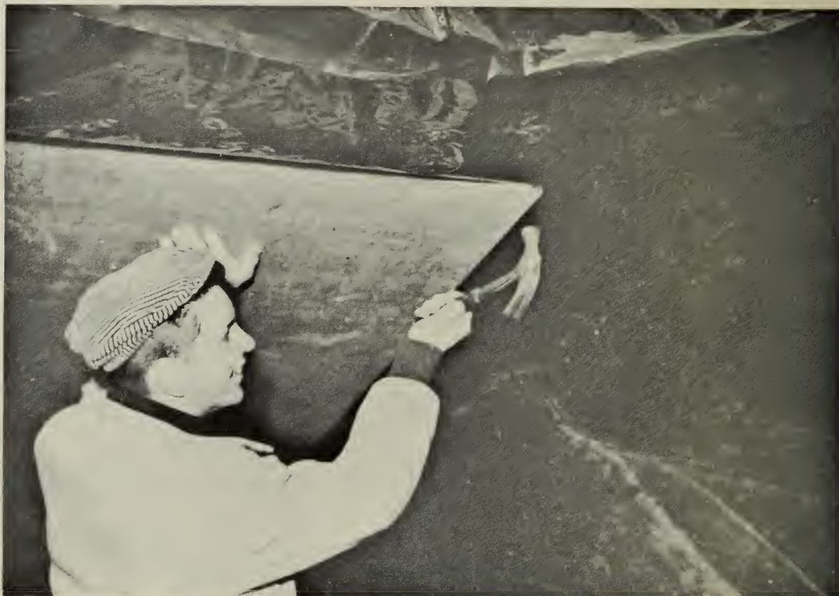
Figure 3. Installing an insulated ceiling in a pig barn. The vapor barrier of polyethylene plastic is placed on the warm side of the insulation, between it and the interior sheathing.
