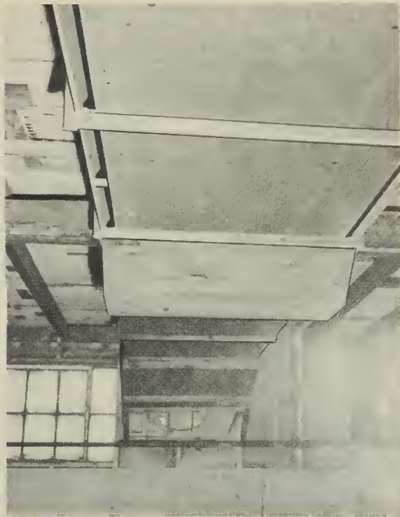
Figure 20. A lateral exhaust duct in a broiler house 60 feet by 365 feet. Note the air inlet slots in the duct.
