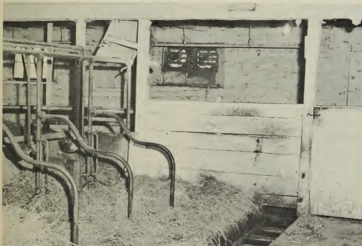
Figure 22. Exhaust fans over calf pens.
