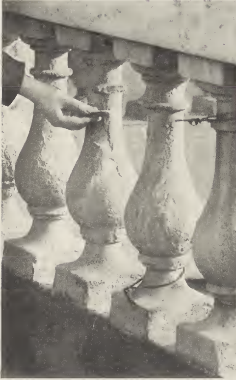
DETAIL OF BALUSTERS—NEW YORK CITY HALL. THE MEREST PRESSURE WOULD BREAK OFF ANY OF THE NECK MOULDINGS AS IT HAS DONE IN THE CASE SHOWN.
