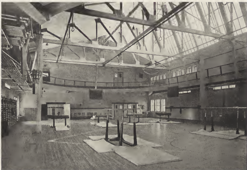
FIG. 17. MAIN GYMNASIUM ON THIRD FLOOR, CENTER SECTION, SHOWING ILLUMINATION THROUGH NORTH SKYLIGHT, THUS AVOIDING SHADOWS; STEEL TRUSSES FIREPROOFED WITH CONCRETE—Y. M. C. A. COLLEGE, CHICAGO.
