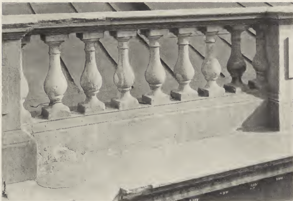
DETAIL OF BALUSTRADE ABOVE ROOF, SHOWING PREVAILING CONDITION OF MARBLE—NEW YORK CITY HALL.
