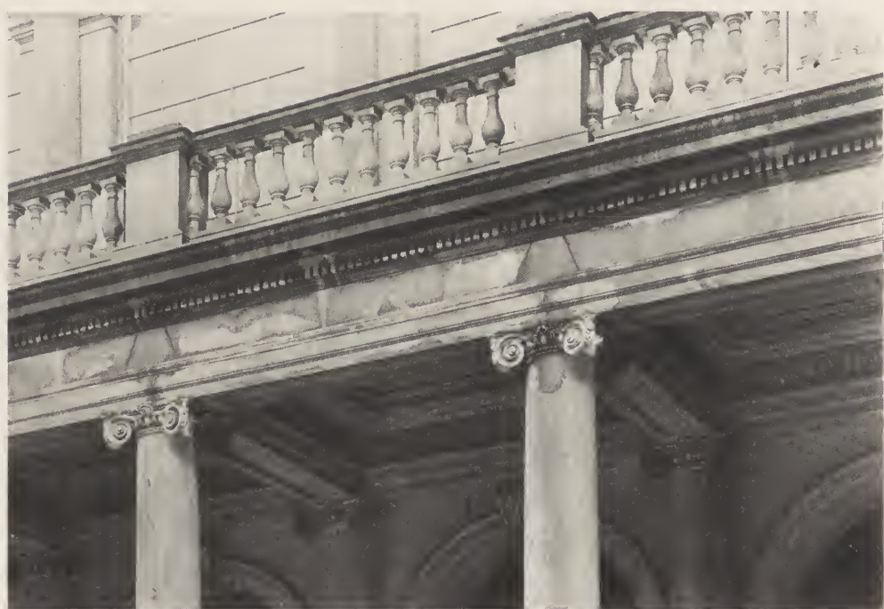
DETAIL AT PORTICO—NEW YORK CITY HALL. COMPARE THE DETAILS OF THE OUTER COLUMN CAPITALS WITH THOSE THAT HAVE BEEN PROTECTED BY THE ROOF.
