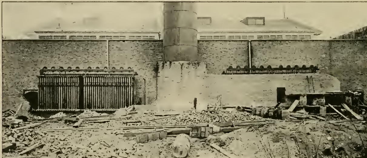
FUEL ECONOMIZER AT WORLD'S FAIR, FROM PHOTOGRAPH TAKEN DURING CONSTRUCTION, SHOWING ONE SET OF PIPES EXPOSED.
