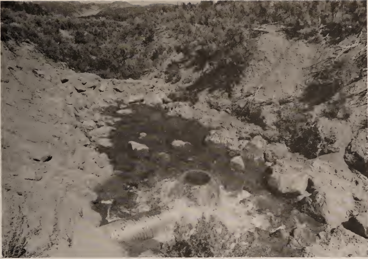
FIGURE 4-18 Energy Dissipation (Erosion Control) System below Lower Pond Discharge Point - East No Name Gulch - August 1979
