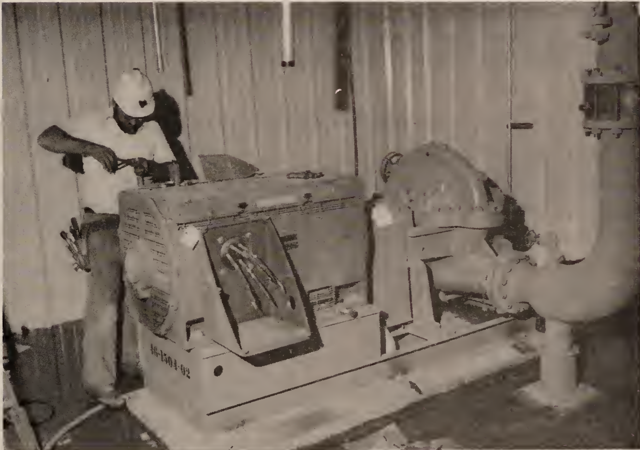
FIGURE 4-19 Pump Inside the Lower Pond Pumphouse - July 1979
