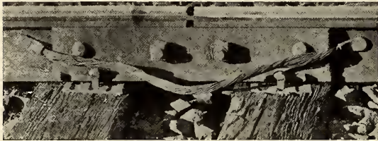
THE "BOND" OF WIRES CONNECTING THE ENDS OF THE RAILS.
