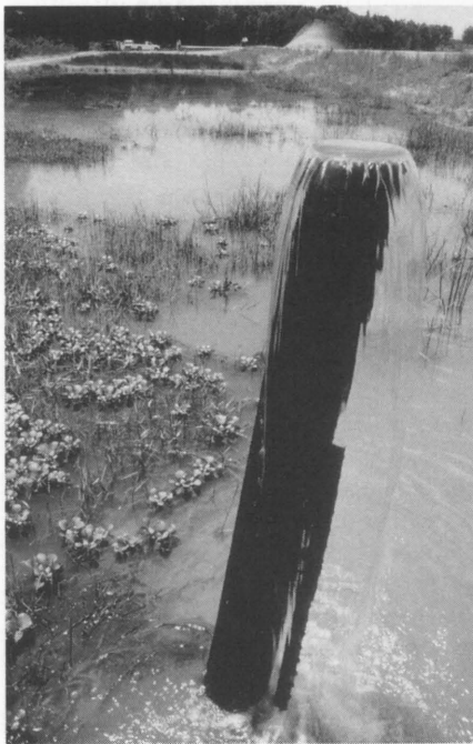
Bottom water from the pond enters wetland filter through a gravity-fed inlet riser.
