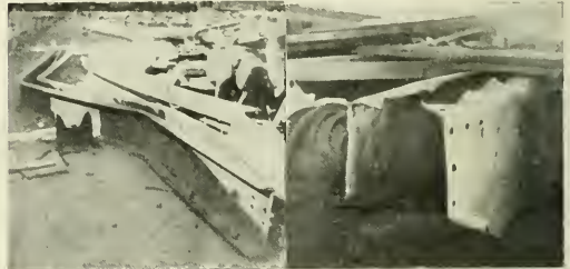
Fig. 4—Weak Center Sills.
