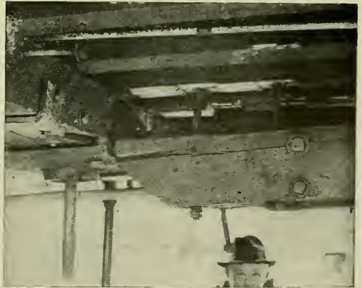
Fig. 2—One of the Common Failures.
