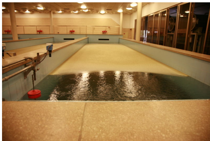
Figure 5: A water purification system at Bret Lake, Switzerland. Contaminants are removed and clean new water is created.
