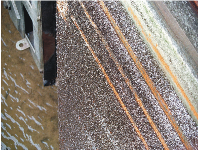
Figure 10: These zebra mussels, an introduced species, colonize most manmade and natural surfaces, including native mussels. Here they have infested the walls of the Arthur V. Ormond Lock, on the Arkansas River. They have caused significant damage to American waterways, locks, and power plants.
