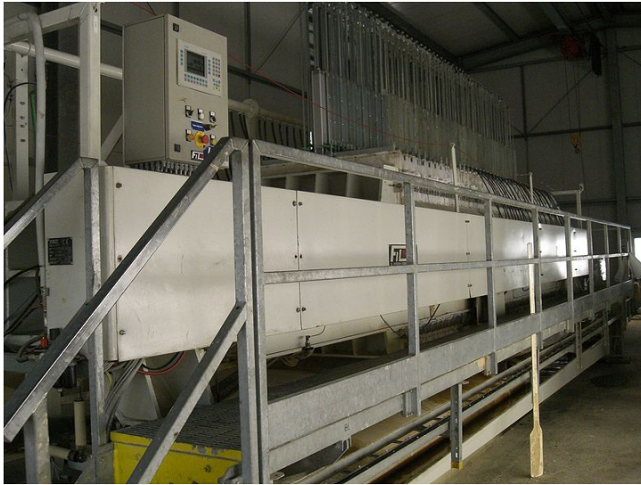
Figure 6: Sand processing Mill, near Provodín, Czech Republic. Water is used to wash mined sand, then is drained into tanks, filtered, and recycled.
