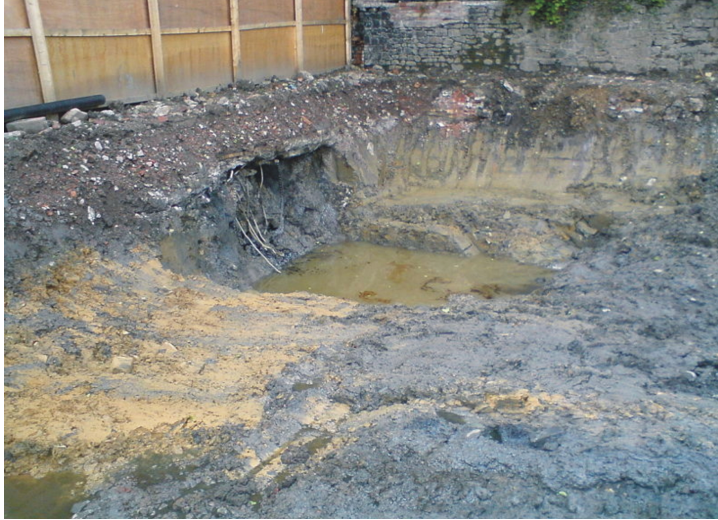
Figure 11: Soil contamination caused by underground storage tanks containing tar.
