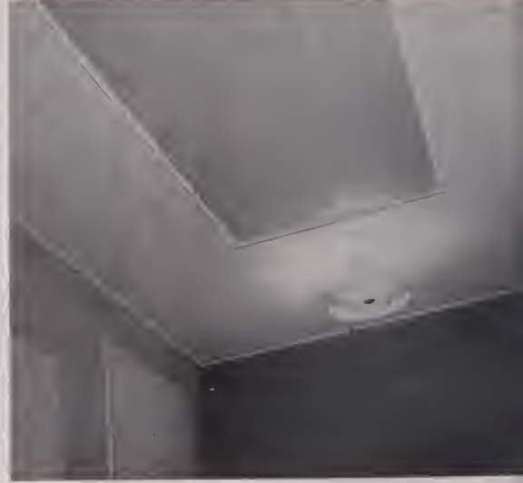
REAR portion of ceiling, showing 4 x 12 foot plywood panel. Better results would be obtained here with a curved panel to minimize sound reflections. —Photos by Aram Peter Margosian
