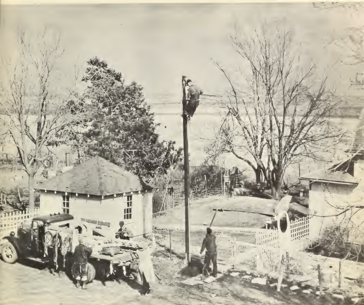
Crews carefully located new poles. This pole does not block gate and will not strike house if wind knocks it down.
