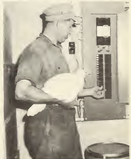
The load center is the nerve center of the modern farm.
