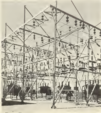
A step-up substation boosts power to 69,000 volts or higher
