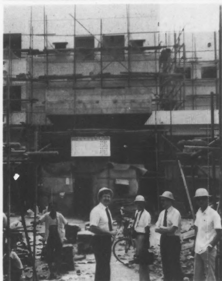
CHENGDU —At construction site for new consulate general is consul general Bill Thomas , second from right, with inspector John Markin , fourth from right.
