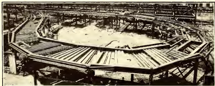
FIG. 1.—VIEW OF DUDLEY STREET TERMINAL, USED IN ADJUSTING A TIME-LIMIT CONTRACT
