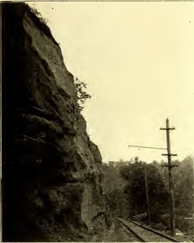
AN EXAMPLE OF THE LARGE ROCK CUTTING REQUIRED ON A 6 DEG. CURVE ONE-HALF MILE LONG
