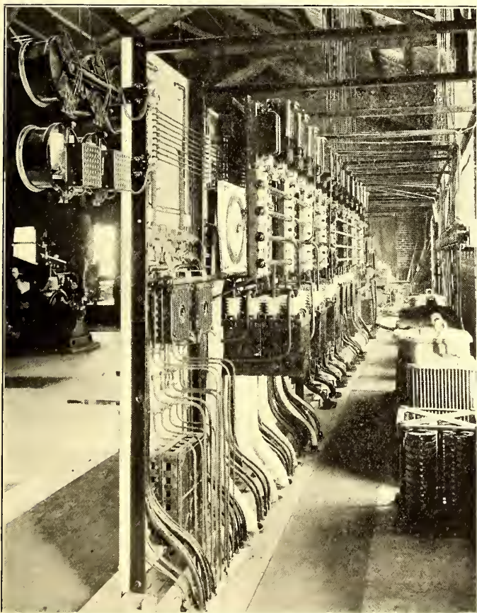
REAR END-ON VIEW OF SWITCHBOARD
