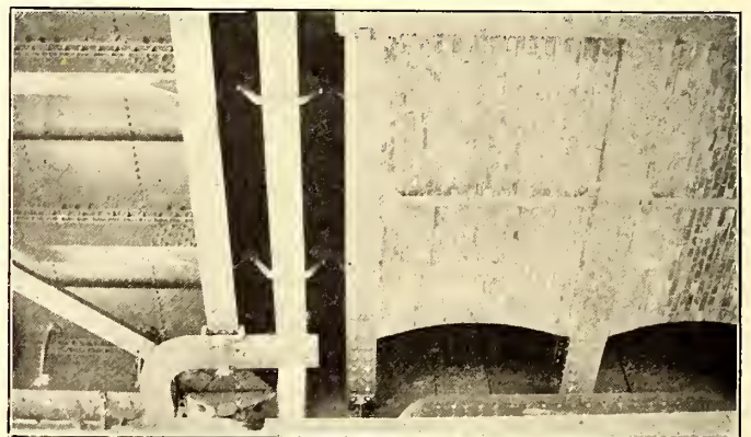
UNDER SIDE OF STEEL-FLOORED BRIDGE TO LEFT, STANDARD BRICK-ARCHED FLOOR TO RIGHT, PARIS
