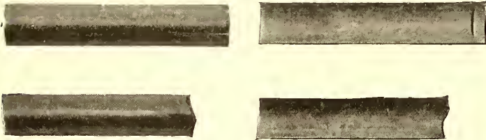
FIG. 4.—WESTINGHOUSE-PARSONS VANE AFTER FIVE AND ONE-HALF YEARS' SERVICE, EIGHTH ROW, LOW-PRESSURE BARREL OF ROTOR, CONVEX AND CONCAVE SIDES
