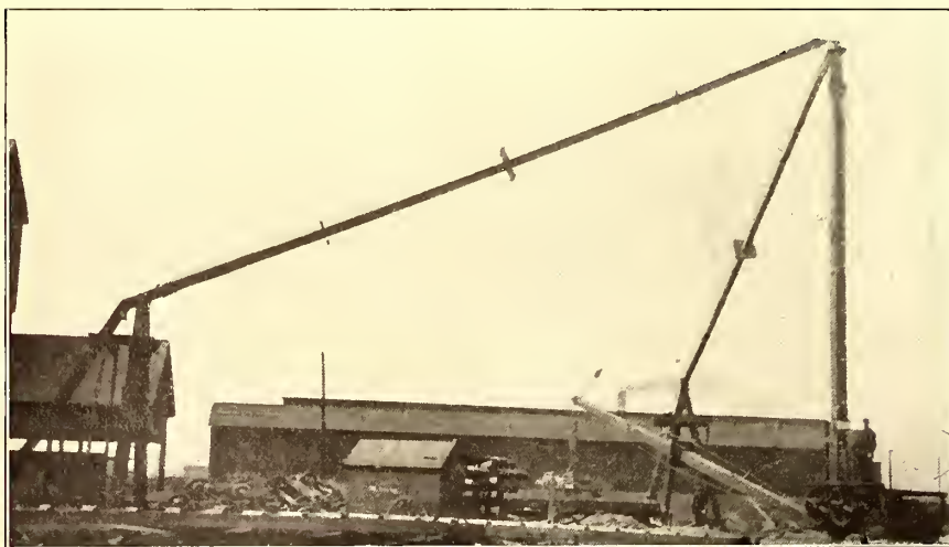
THE MOTOR-DRIVEN DERRICK AT WORK IN THE YARDS OF THE DETROIT UNITED RAILWAY
