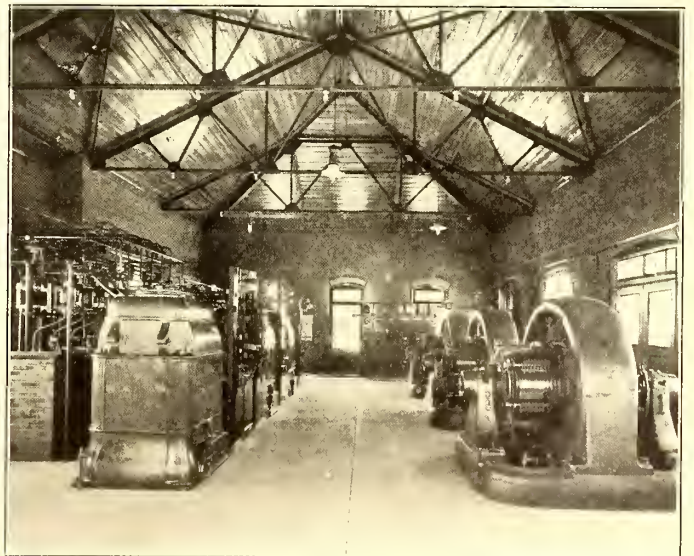
INTERIOR BRIDGEWATER SUB-STATION
