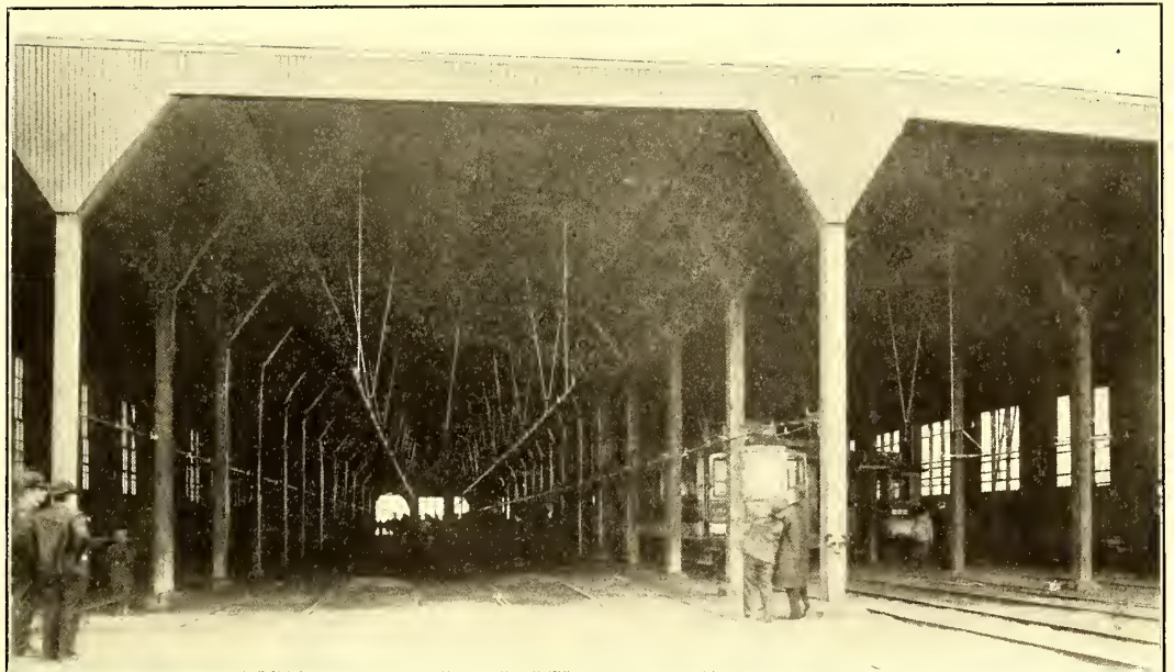
INTERIOR OF CAR HOUSE FROM SOUTH END, SHOWING SIDE AND ROOF SPRINKLERS
