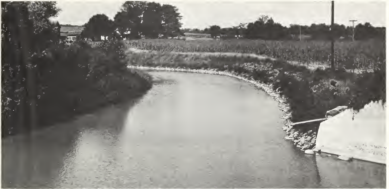
With the bank sloped and the lower part protected by rock riprap, this section of Buffalo Creek in New York is being stabilized with vegetation. The costly effects of streambank erosion are illustrated (opposite page) on a farm in Louisiana where the Red River cuts away a strip of land 200 feet wide in 3 weeks.
