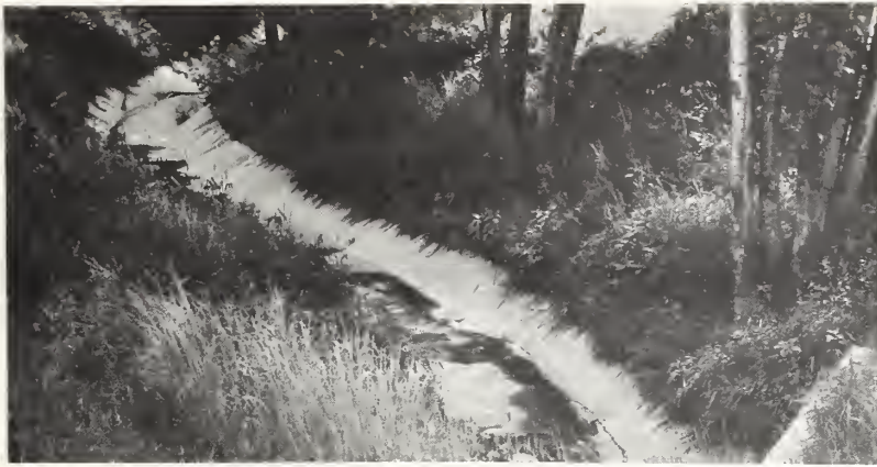
A concrete-lined drainage way (above). While grading is still underway (right), fescue protects soil.
