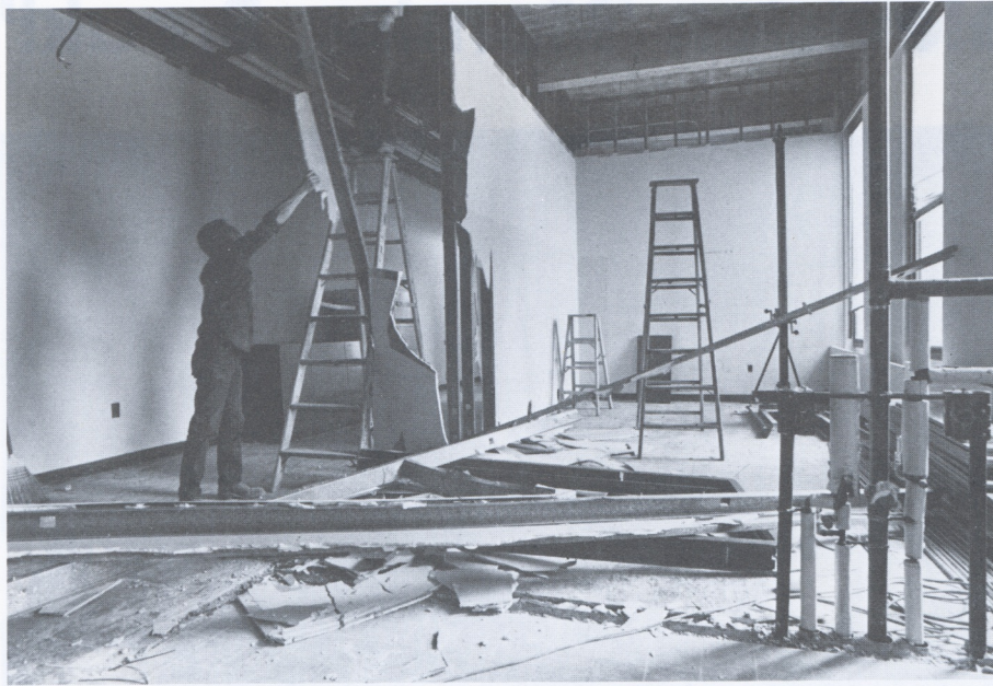
Workmen tear down walls as the first step in enlarging the School of Food, Hotel and Tourism Management's on-campus restaurant facility.
