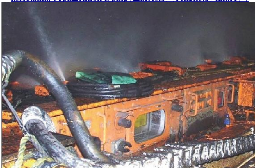
Figure 3-10.—Directional sprays mounted on face side of shearer body.
