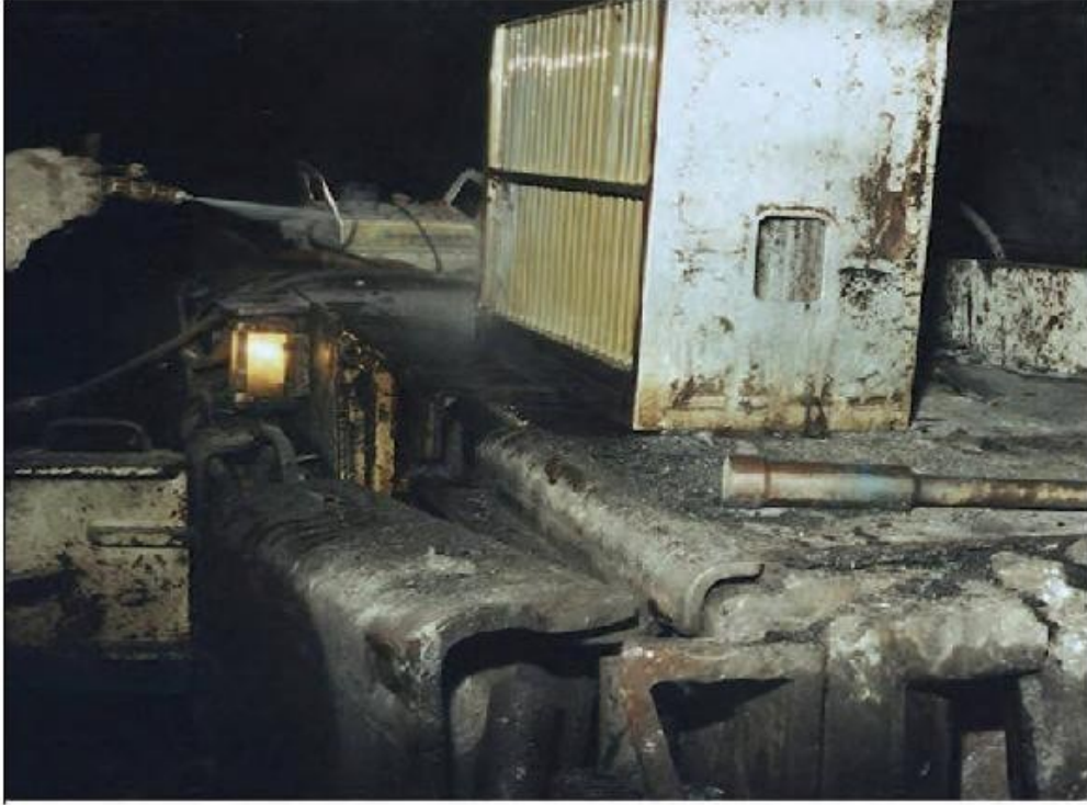
Figure 4-8.—Cleaning the demister with a water nozzle.
