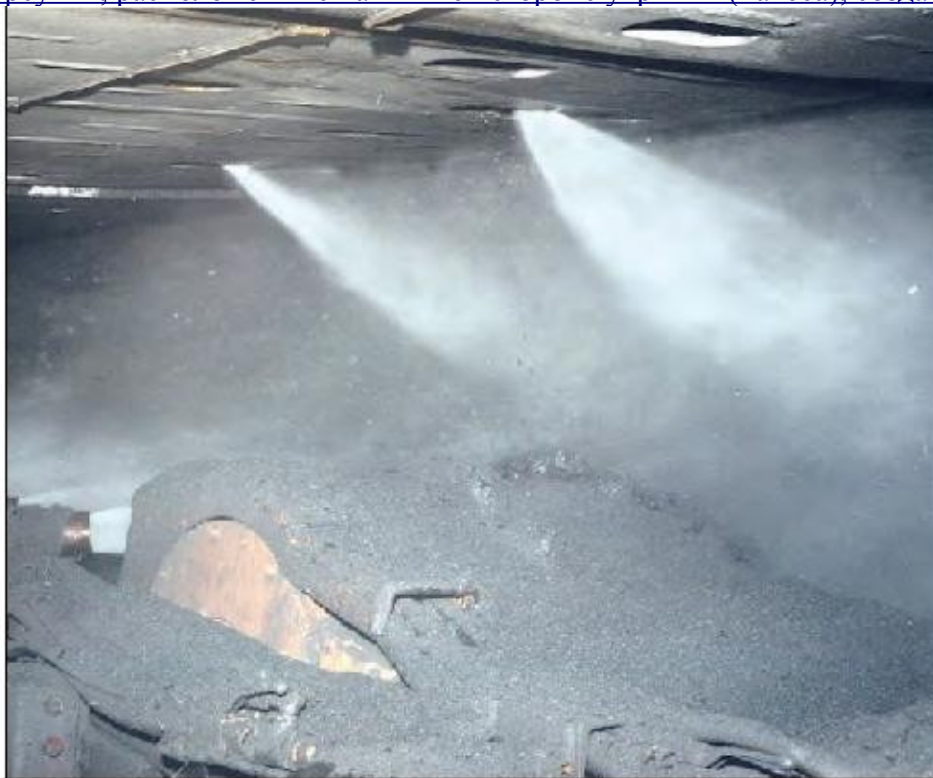
Figure 3-15.—Shield sprays located on the underside of the canopy.
