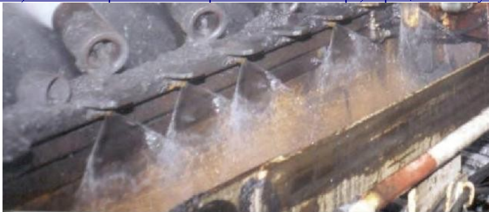
Figure 3-9.—Headgate splitter arm with flat-fan sprays mounted on gob side of belting.
