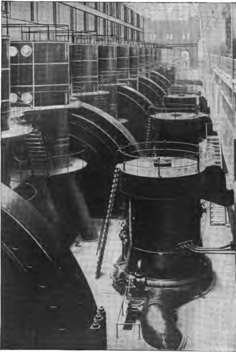
FIG. 181c. Steam Turbines taking the Exhaust from Large Reciprocating Engines.
