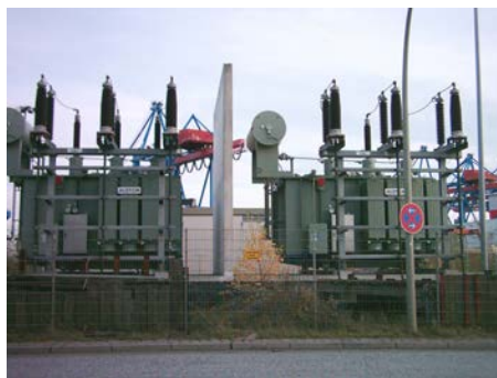
Figure 20.19 Power is distributed over large distances at high voltage to reduce power loss in the transmission lines. The voltages generated at the power plant are stepped up by passive devices called transformers (see Transformers ) to 330,000 volts (or more in some places worldwide). At the point of use, the transformers reduce the voltage transmitted for safe residential and commercial use. (Credit: GeorgHH, Wikimedia Commons)
