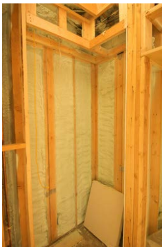
Figure 14.13 Insulation is used to limit the conduction of heat from the inside to the outside (in winters) and from the outside to the inside (in summers). (credit: Giles Douglas)
