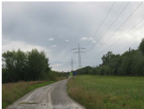
Figure 24.10 This high-voltage traction power line running to Eutingen Railway Substation in Germany radiates electromagnetic waves with very long wavelengths. (credit: Zonk43, Wikimedia Commons)
