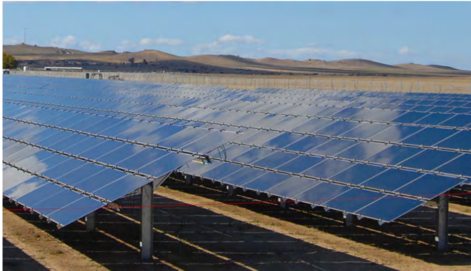
Figure 8.16 Solar cell arrays found in a sunny area converting the solar energy into stored electrical energy. (credit: Sarah Swenty)
