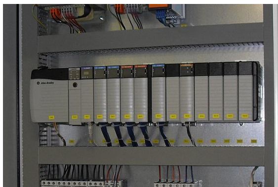
Allen-Bradley PLC installed in a control panel
