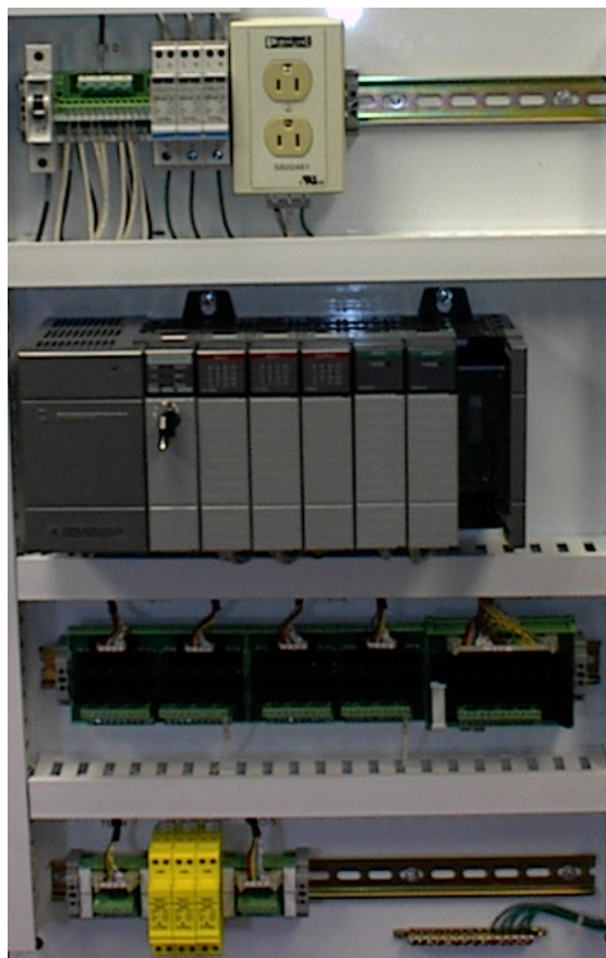
Control panel with PLC (grey elements in the center). The unit consists of separate elements, from left to right; power supply, controller, relay units for in- and output
