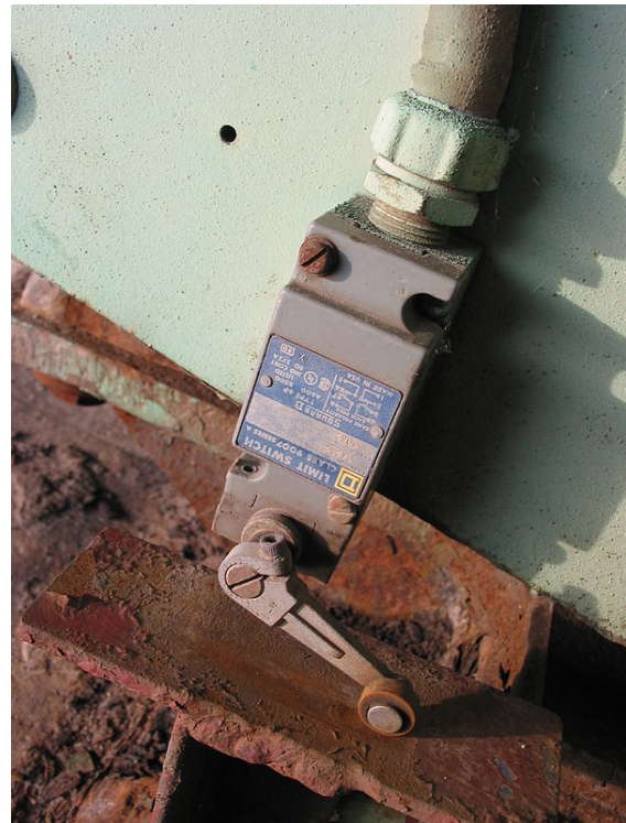
A limit switch mounted on a moving part of a bridge.
