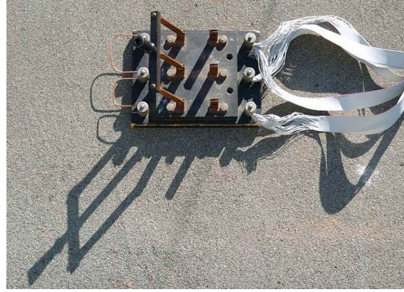
Triple-pole single-throw (TPST or 3PST) knife switch used to short the windings of a 3-phase wind turbine for braking purposes. Here the switch is shown in the open position.
