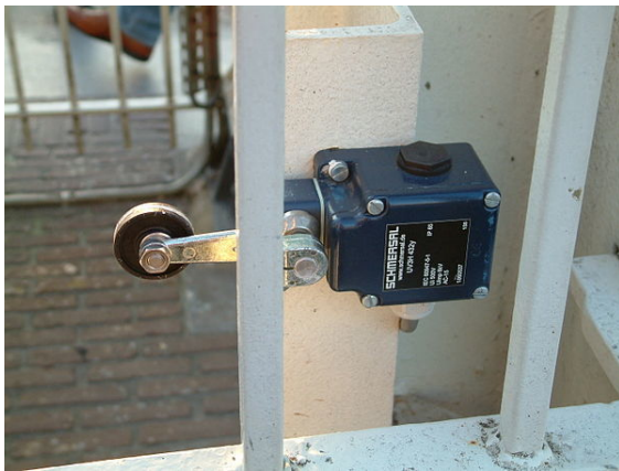
A limit switch with a roller-lever operator; this is installed on a gate on a canal lock, and indicates the position of a gate to a control system.
